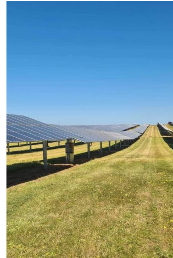
Solar farm in operation
