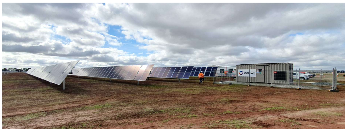
Hybrid Power System located at Quorn Park Solar Hybrid project, May 2025.
