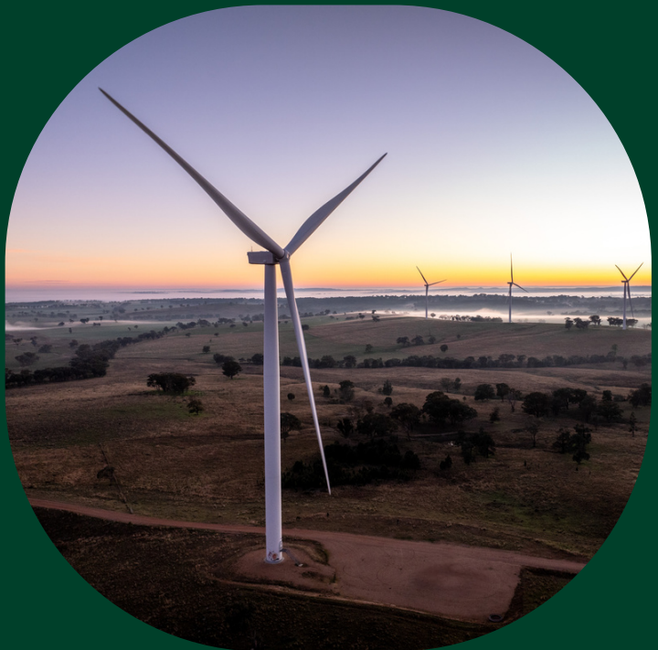
Bodangora Wind Farm – T16 in the foreground, with T28, T29 and T30 in the background
